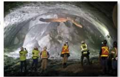
Workmen take photos inside the Caldecott Tunnel where the boring from the two sides finally broke through.
